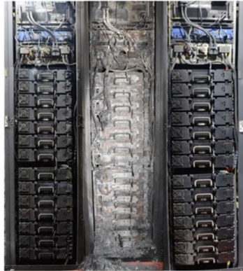
Rack 17 Rack 15 Rack 13
