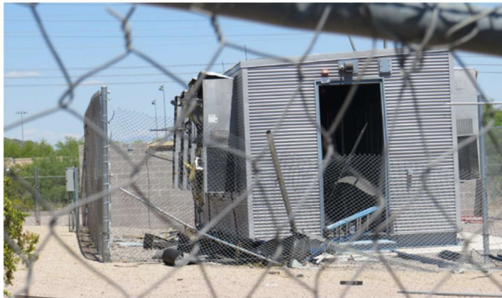
Figure 4: The 2 MWh McMicken (Arizona) BESS after the explosion on 19 April 2019
